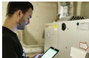
Mobile and BIM based maintenance.
